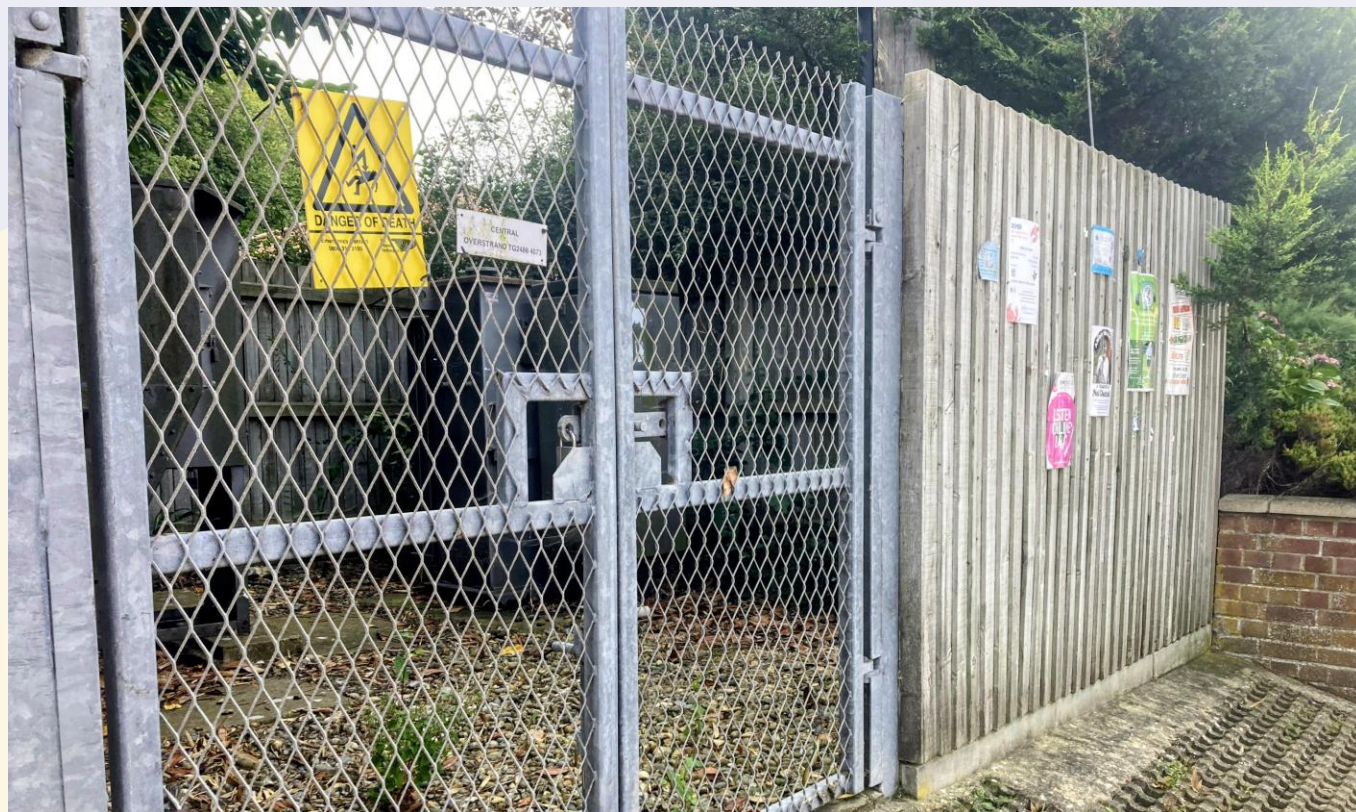
Figure 21 (Top): View of Highstreet looking west. Figure 22 (Bottom): Electricity substation in Overstrand. Images taken by JBA Consulting, September 2025.
