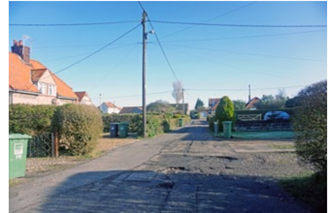
Poor surfacing of The Fairhaven
