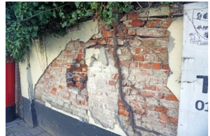
Wall in poor condition on the High Street
