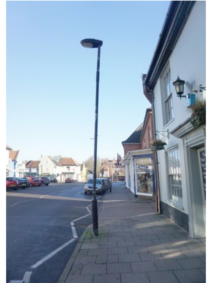
Basic modern lamppost which had been damaged and is now leaning
