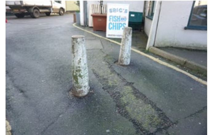
Unattractive concrete bollards with peeling paint
