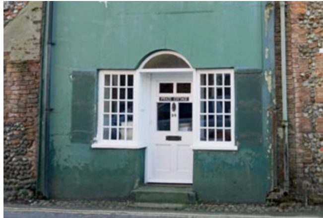
Poor condition of paintwork
