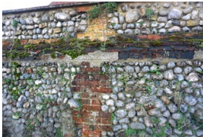
Wall with vegetation growth and patches of cement pointing, indicating damp and poor condition
