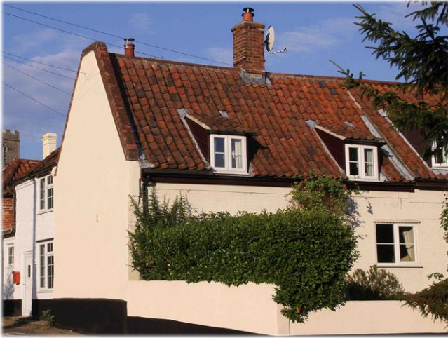
5. End of terrace forming entrance to Great Yard showing wedge dormer windows in pitched roof
