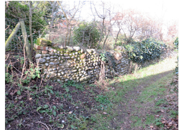
A poorly maintained wall that has started to suffer substantial loss
