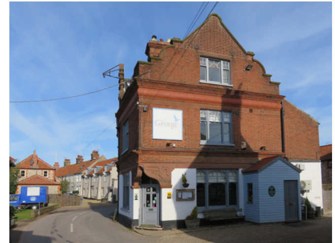
The combination of air conditioning unit, lights, alarm, junction box and signs create a cluttered appearance
