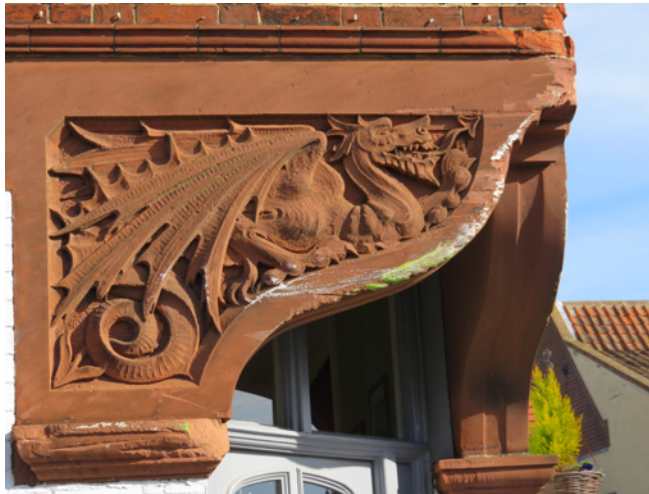
The terracotta dragon at the corner of The George shows evidence of damage from vehicles
