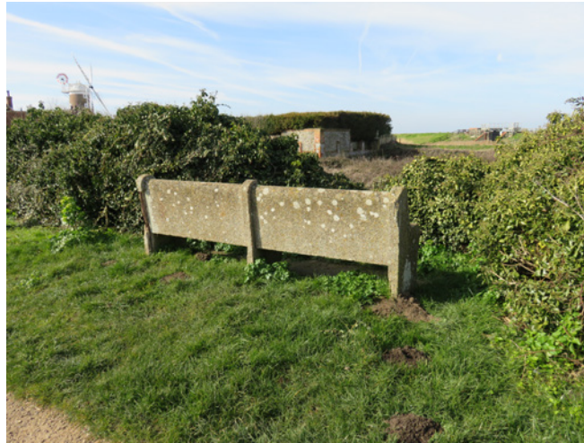
This reinforced concrete seat on the Coast Road is in poor condition and detracts from the quality of the area
