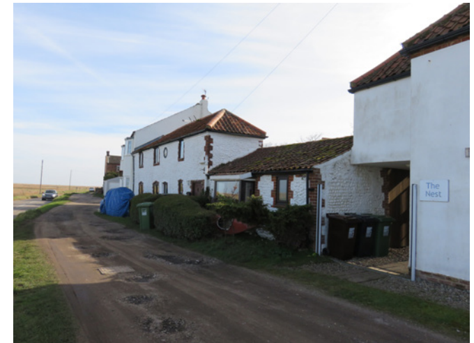
Potholed tracks detract from the setting of the buildings and are a potential source of injury for pedestrians
