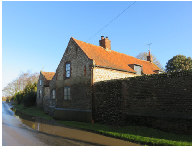
Green Farmhouse and boundary wall is soaked by passing cars driving through the water collected in a dip in the road
