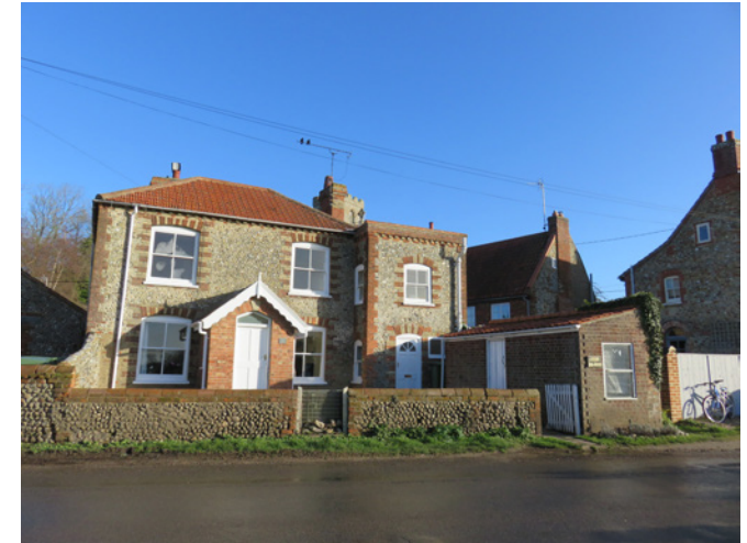
The boundary wall is in poor condition and spattered with mud. The gate should also be reinstated
