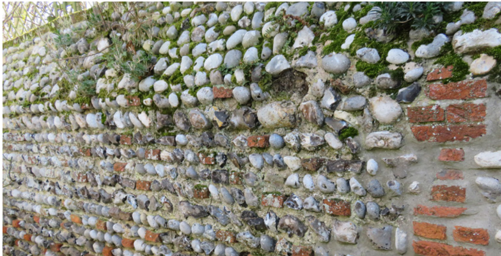
Flints will fall out of walls that are not well maintained. Vegetation growth causes damage to walls. Poor quality cement repairs affect the appearance of walls, especially where they cover the edges of the brick
