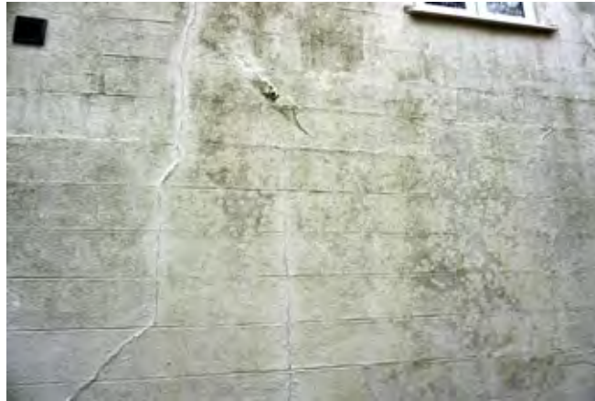
Cracked render and dirty paintwork
