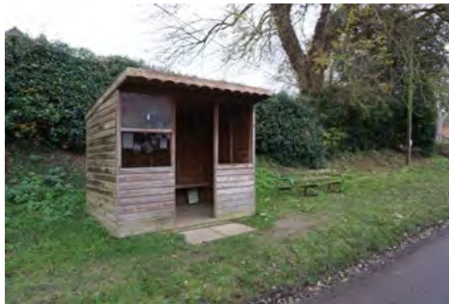
Bus shelter in poor decorative condition
