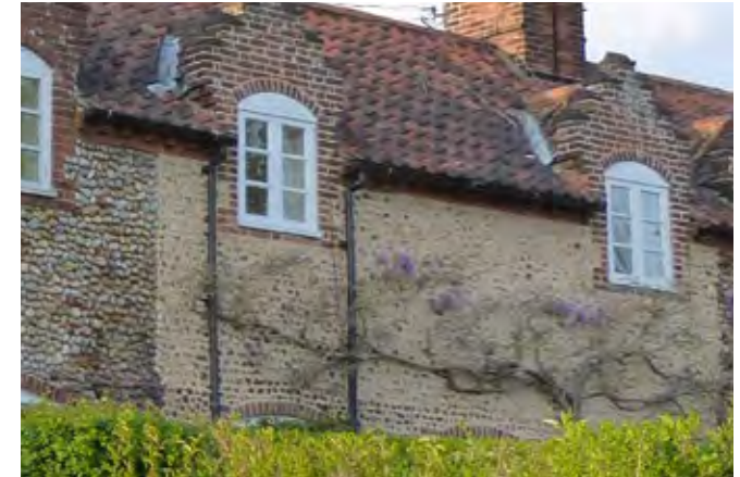
Poor pointing which obscures the flintwork on the wall
