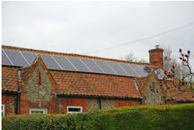
Prominent solar panels disrupt the visual appearance of the historic building
